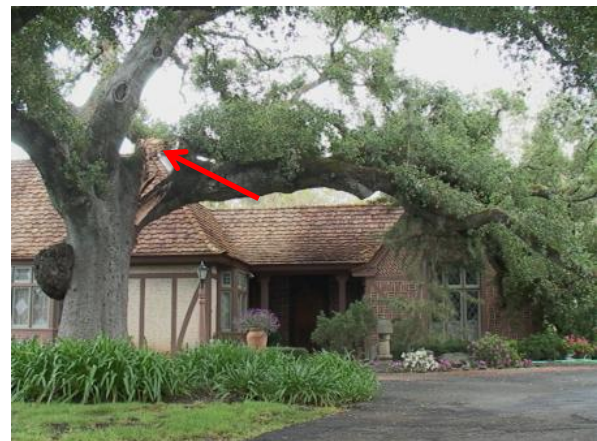
Fig. 2. Branch failures occur at the point of attachment (arrow) or along the branch. Photo courtesy of B. Glen.
