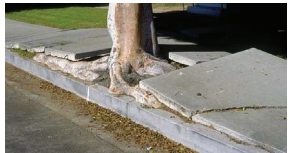
The right tree in the right place can prevent infrastructure damage. Photo Courtesy: PasadenaNow
